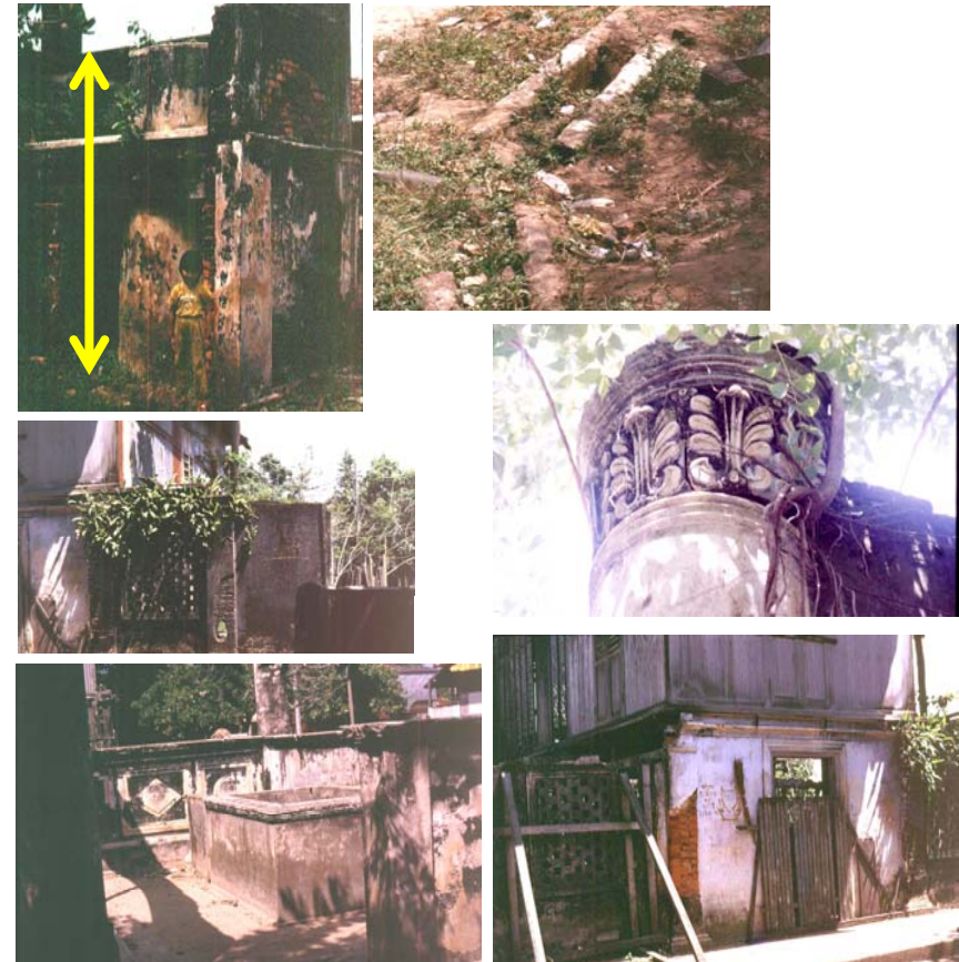
Fig. 15 - Condition of Kota Duyung before it was restored: the elevated indoor well (top left), physical traces of surface drainage (top right), part of the wall and Rumah Bujang overgrown with ivy (centre left), the round pillar with its characteristic capital (centre right), pool to store water placed at house front for ablution and washing feet (bottom left), half-hearted attempt to braced part of collapsing wall (bottom right).
