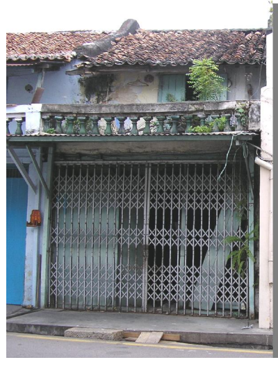
Fig.6: A dilapidated old shophouse
